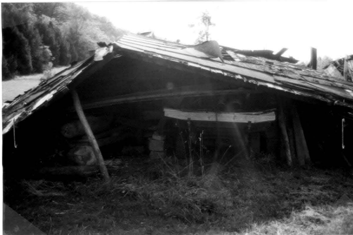
Photo #16 Collapsed structure "sawmill"
