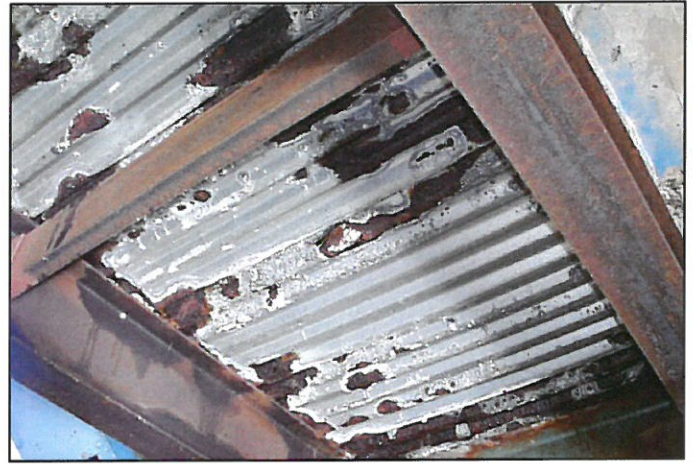
Detail View Showing Deterioration to Underside of Deck
