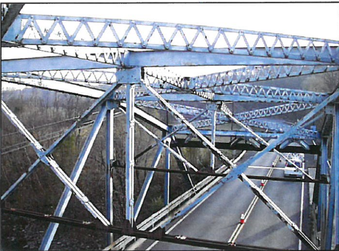
Detail View of Deteriorated Cross Beams
