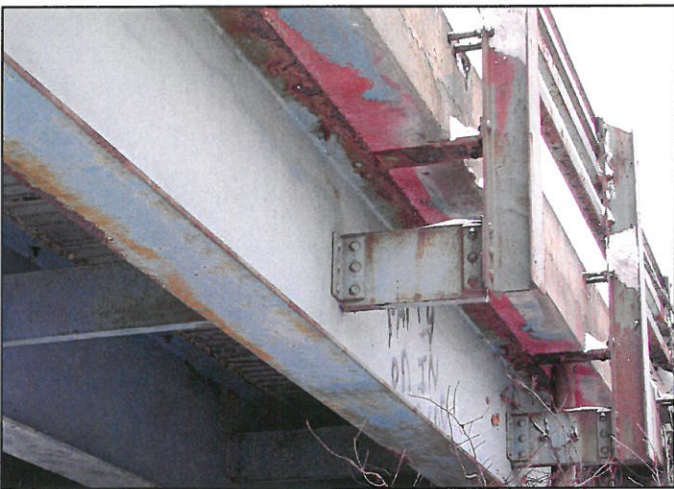
Detail View of Deteriorated Railing Anchors
