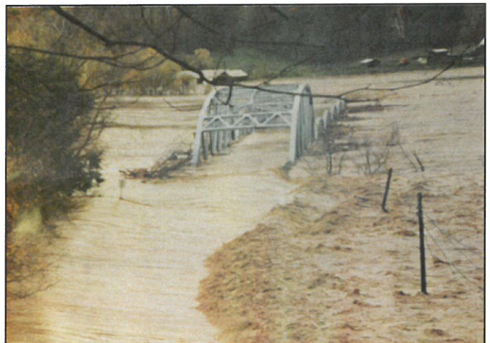
View of Inundated Romney Bridge during 1985 Flood
