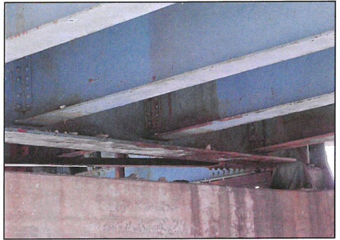
Detail View Showing Deterioration to Support Beams
