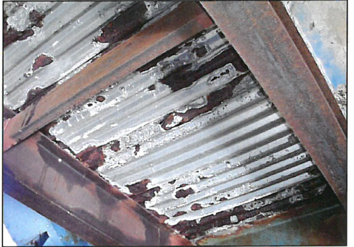
Detail View of Deteriorated Replacement Deck Supports
