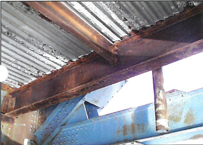
Detail View of Deteriorating Beams
