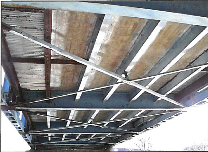
Detail View of Deck Repairs—Underside
