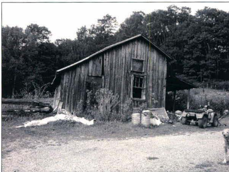
Photograph of a dependency (Feature H) found in association with the Double-Pile Cottage
