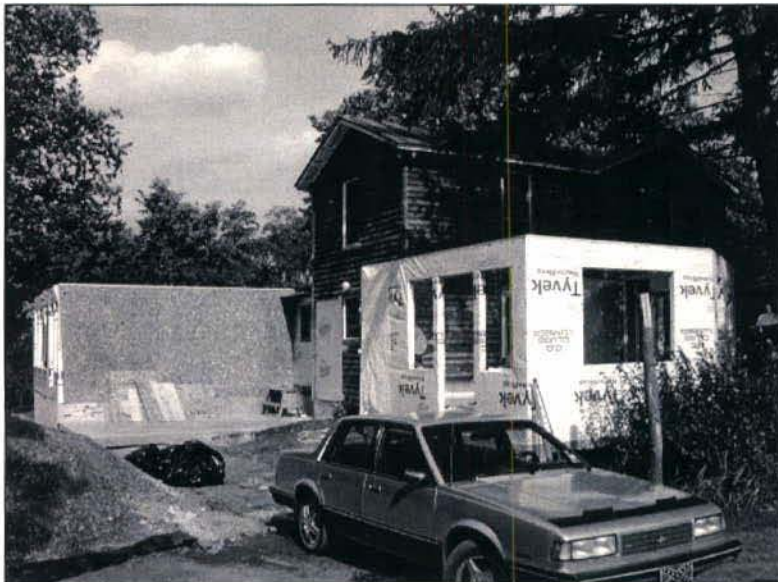
Photograph of the ongoing renovations at the Judy Harman House, facing southeast.
